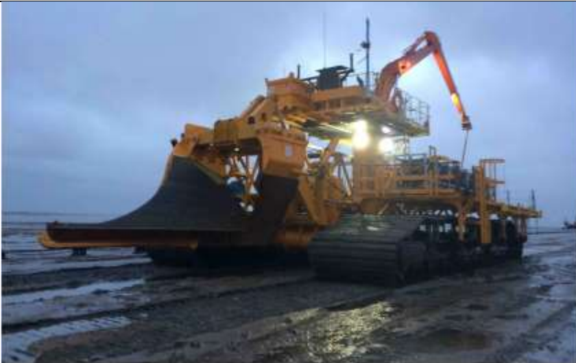
View from the Sea defence at Sutton Bridge of the work barges and tugs positioning the cable laying barge into position.
