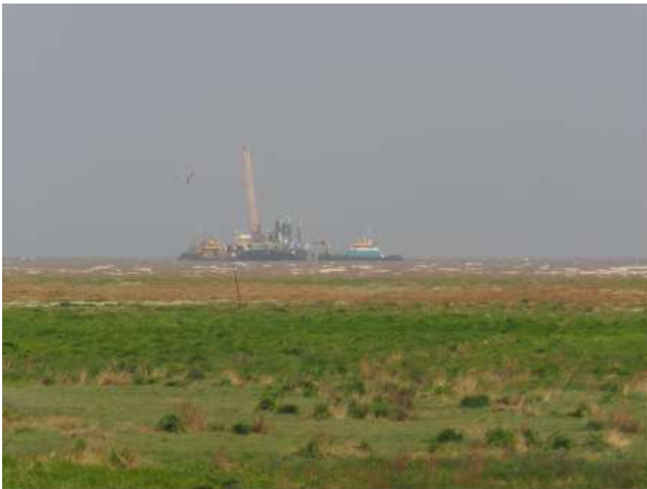
The First section of cable has now successfully been laid throughout the Port of Wisbech area of Jurisdiction. The plans are currently still on track to install two cables this year.
